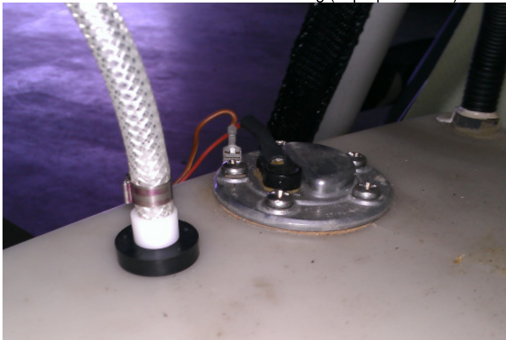
Photo 8: Return line with rubber bushing (unprepared tank)
